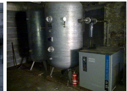
Compressor air tanks and dryer
